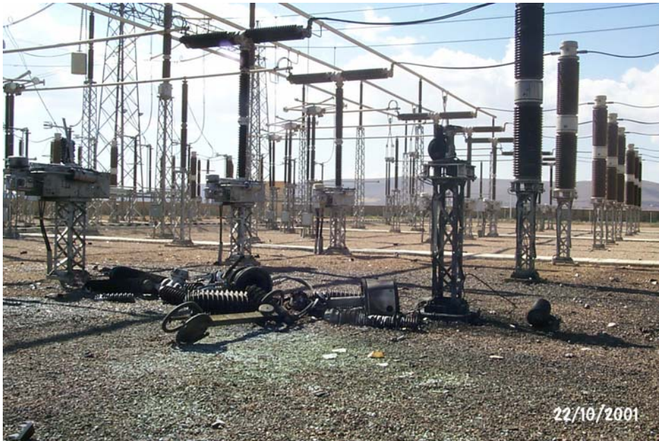
Figure 5-1- Damaged bay in a high voltage outdoor substation
