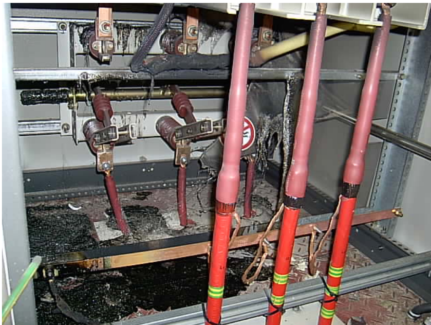
Figure 5-2- Damaged cubic in a medium voltage metal-clad switchgear
